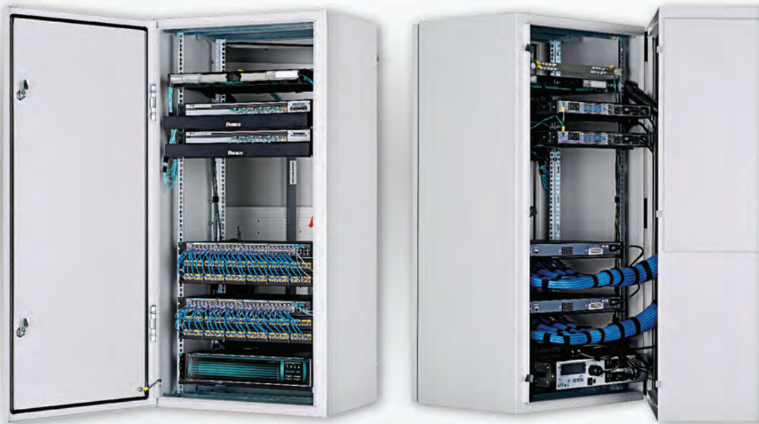
IDF Installation Example
