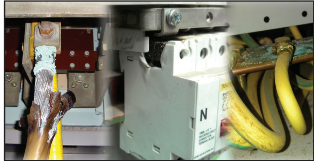
Fig 16: Typical faults that can be prevented by low resistance testing
