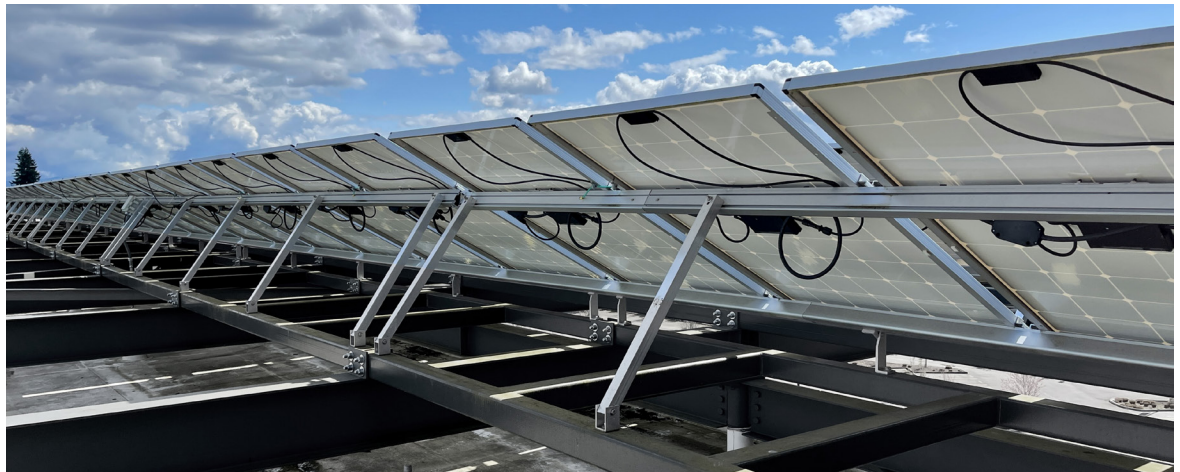
If you work on PV panels, you should know how to work with a non-load break rated disconnect.
