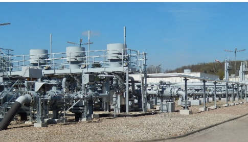
Underground natural gas storage facility in Empelde near Hannover, Germany. Gerd Fahrenforst/CC BY 3.0
