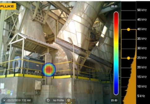
Air leaks detected in a cement plant with the ii900 Sonic Industrial Imager.
