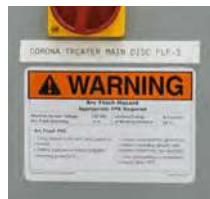
Arc Flash Panel Labels
