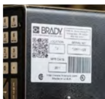
Panel Rating Plate Materials
