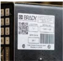
Panel Rating Plate Materials
