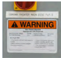
Arc Flash Panel Labels
