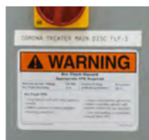
Arc Flash Panel Labels
