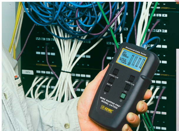
Model CA7028 used to locate and test a cable from the patch panel to an office a few hundred feet away.
