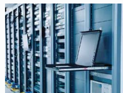
Control Room/ Data Center
