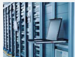
Control Room/ Data Center
