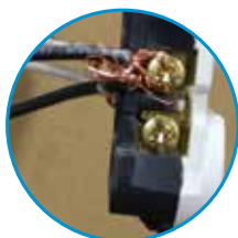
Improper stranded wire connection.
