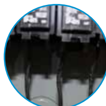
Improperly torqued circuit breaker lugs.
