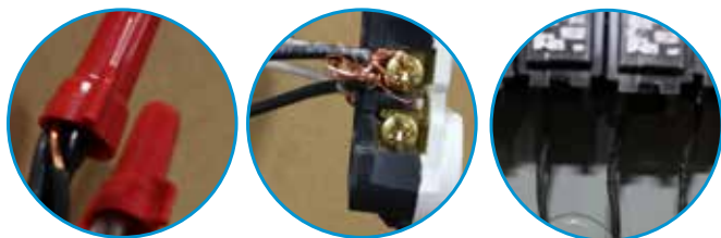
Improper solid wire connection. Improper stranded wire connection. Improperly torqued circuit breaker lugs.
