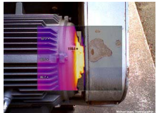
Overheating motor with winding issue.
