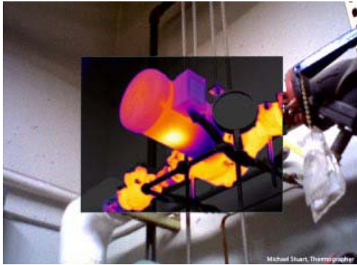
Bearing problem on a drive motor.
