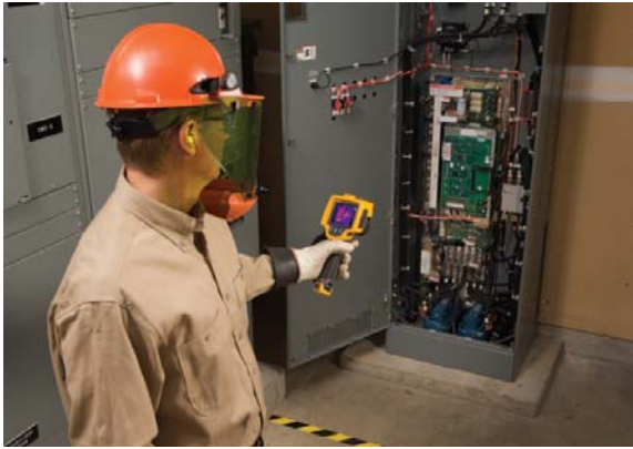
Inspection with the Fluke Ti32 Thermal Imager can reveal defective components and maintenance issues, such as energy-wasting loose connections.
