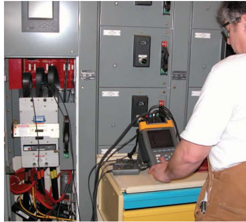
Maintenance Electrical Specialist Mark Newport using a Fluke 434 Power Quality Analyzer to measure, trend, and document the power factor and harmonics correction provided by the plant's new power correction system.
